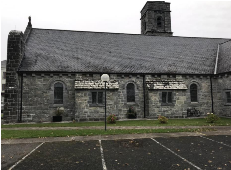
Cill Einde, An Spideal – repairs to South façade pointing & to rainwater goods
