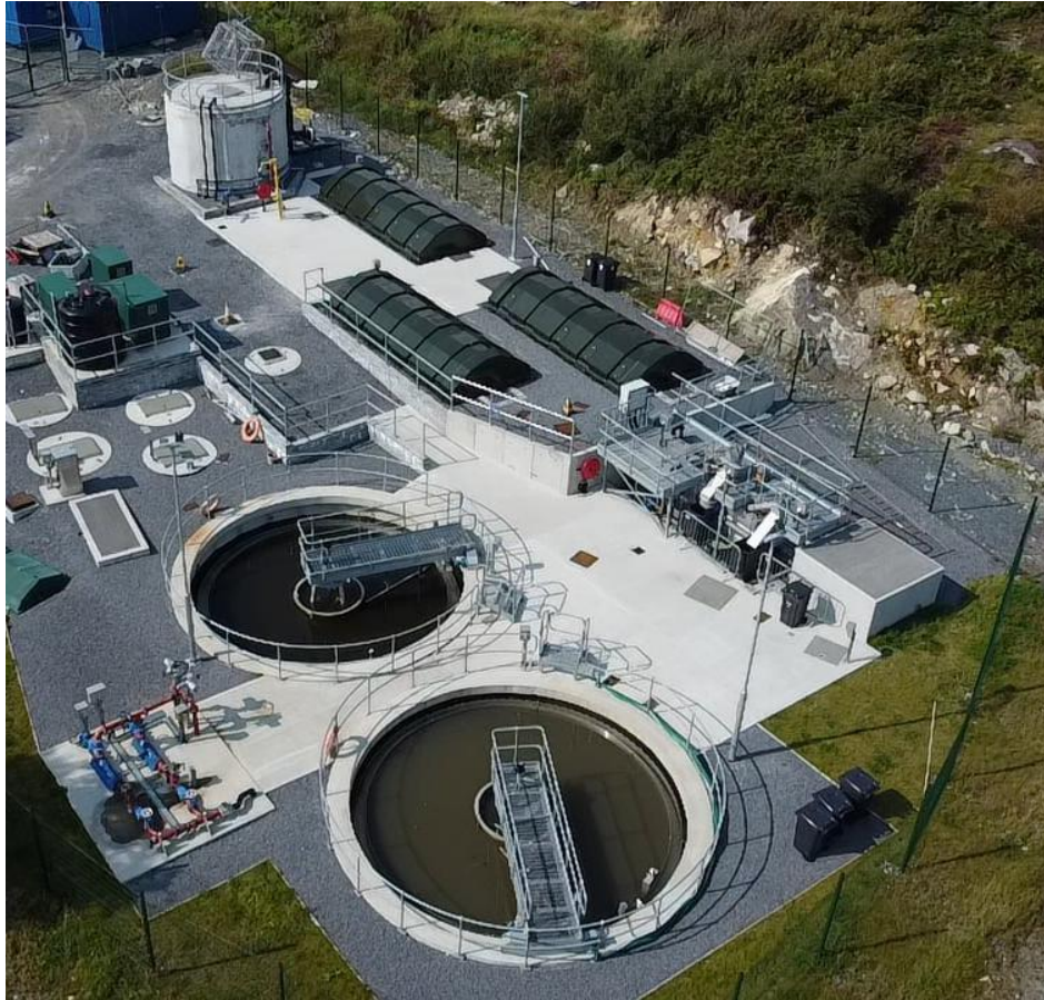
Spiddal Wastewater Treatment Plant
